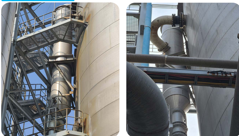
▶ Methane gas storage
