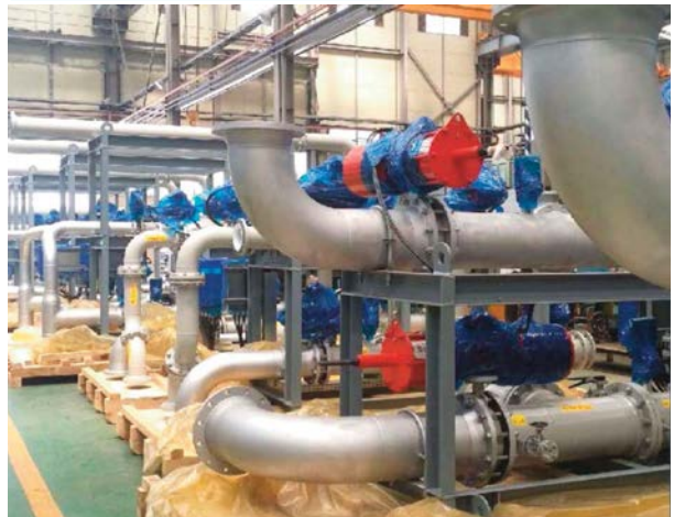
Front Pipe Skid
